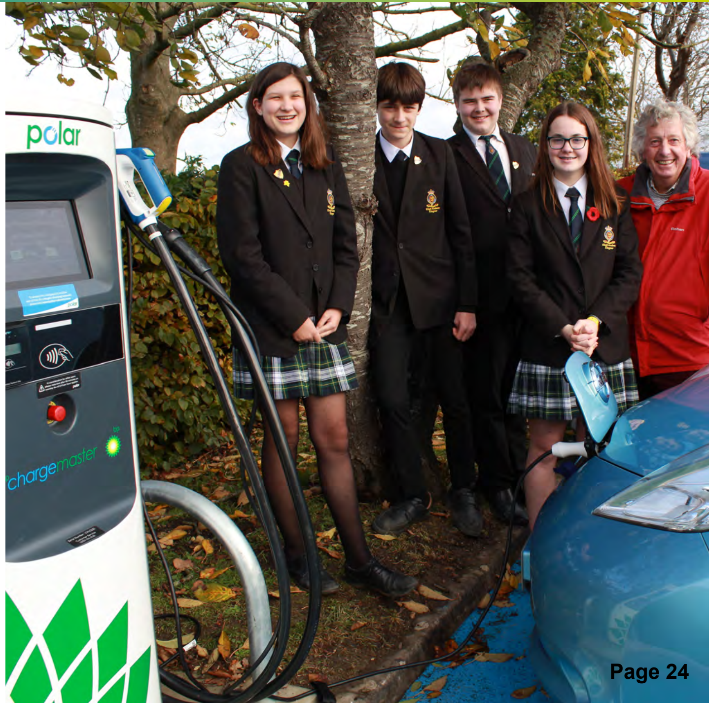
RIGHT Rapid Charger installed at Kings Academy, Ringmer
