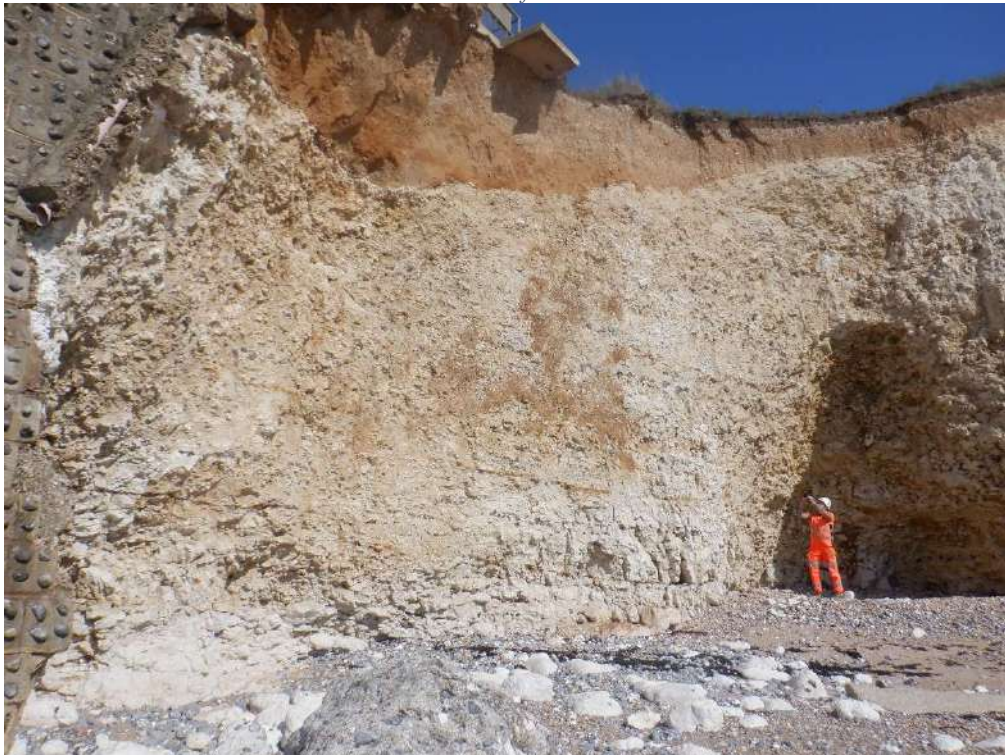
Photograph 2 - Showing eroded section of cliff below steps, looking north and undercutting
