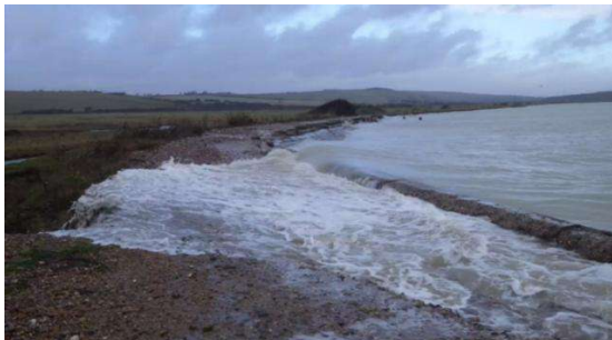
Fig 1. Breaching of flood embankment (2014)
