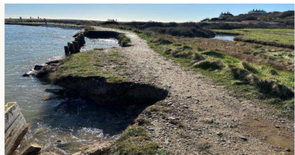
Fig 2. Erosion of flood embankment (2024)
