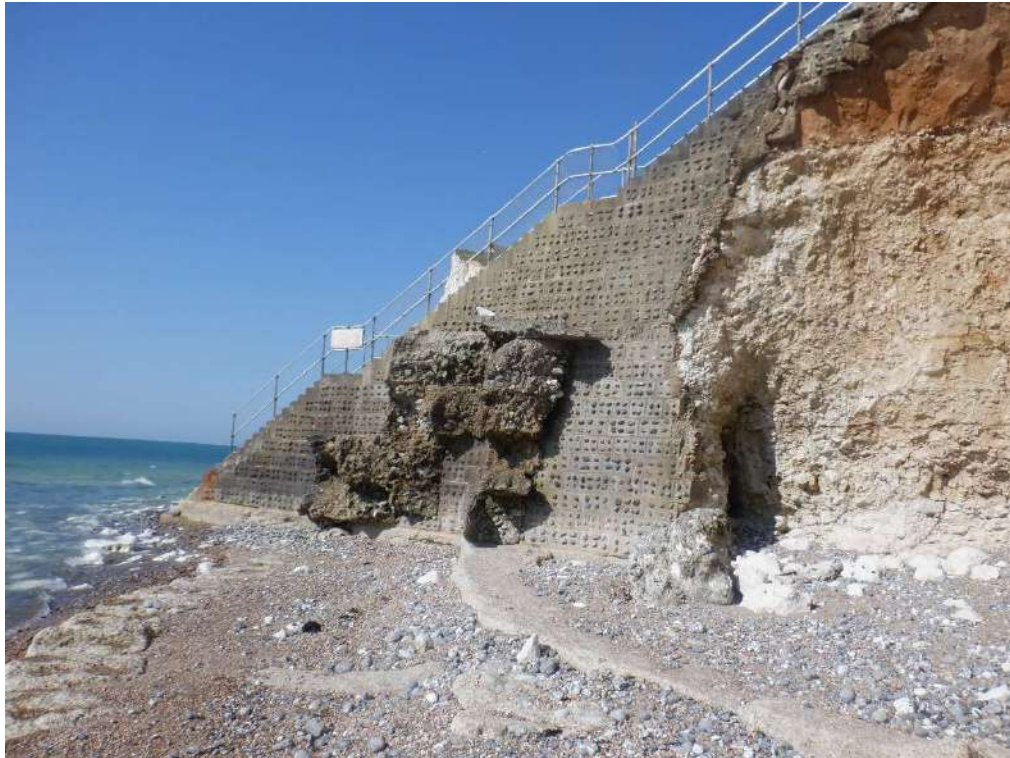
Photograph 3 – Indicating east elevation of cliff steps, note junction to suspected historical coastal defence now lost and erosion behind weathering wall.
