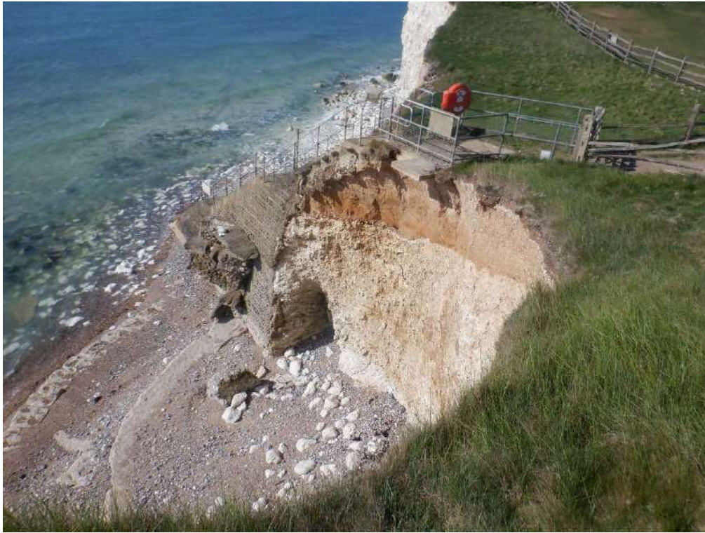
Photograph 1 – Indicating general overview of steps from cliff level, looking southwest. Note undermining, support from near vertical topsoil underlain by weathered chalk, loss of weathering wall and suspected arching foundations to historical coastal defences.
